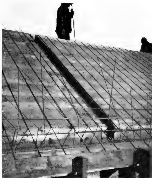
7—The Forms for the Roof, Showing the Reinforcement Rods in Position Ready for the Concrete
